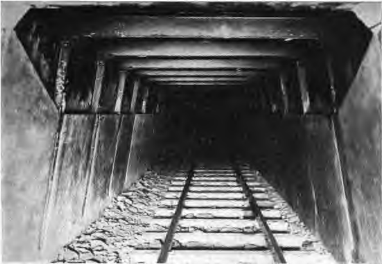
Fig. 8. Steel Gangway Supports, Style F, Allport Coal Co., Barnesboro, Pa.
